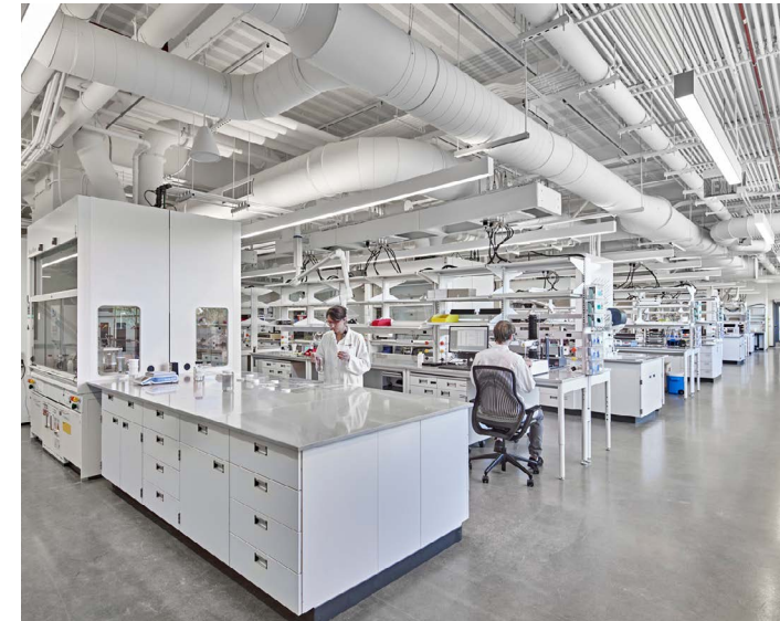
At the Wacker Innovation Center and Regional HQ, their laboratory infrastructure of HVAC, electrical, and plumbing is modularized and highly adaptive for future reconfigurations of their research environment.
